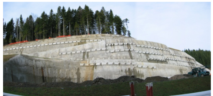
Picture 2: The picture shows permanent reinforcement of the slope before the construction of oil-tanks. The protection is performed by five armored concrete beams tied up with permanent prestressed geotechnical anchors. Immediately after the excavation the slope was simultaneously sprayed with shotcrete in thickness d \approx 0,2 m over heavy reinforcement meshes.
